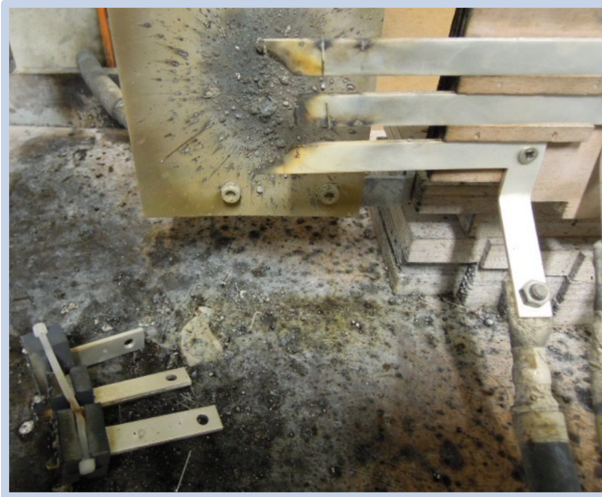
Example of busbars after arcing Zodiac experiments
